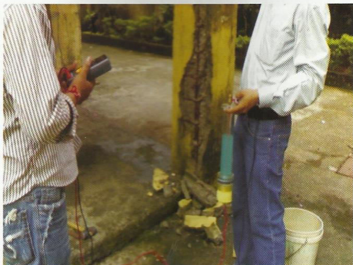
Figure 4. Testing on reinforcement steel to know extent of corrosion and rebar continuity by Half-cell Potential Meter
