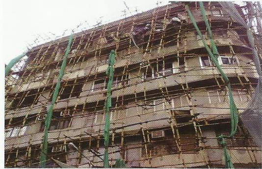
Figure 9. Continuous sunshade being provided
