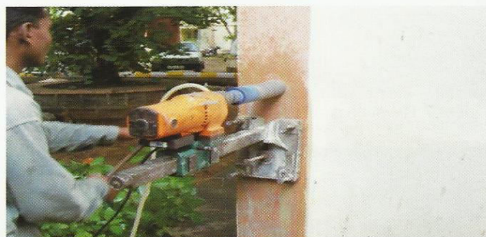
Figure 5. Core cutting of concrete to test chemical properties and compressive strength at lab
